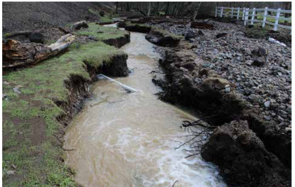
A critical water pipe exposed when a stream changed course during a flood in Cowlitz County.
