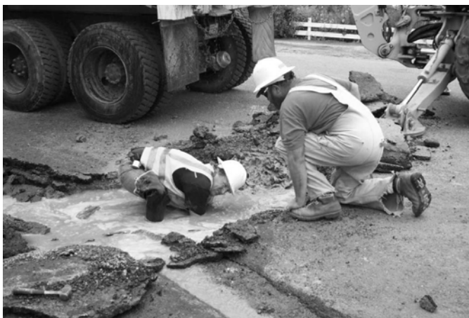
Mike Carlstrom, Tacoma Water construction inspector, tackles a distribution system leak. Tacoma Public Utilities Photo
